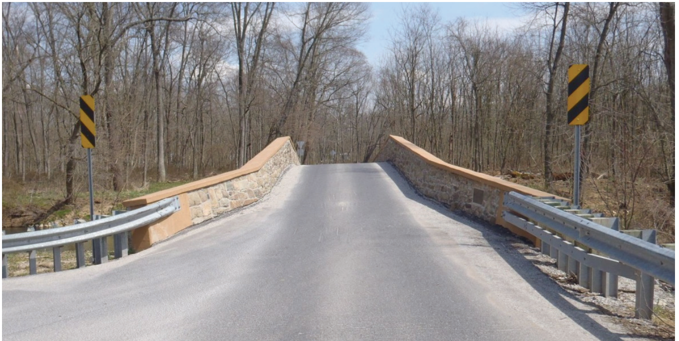
The hazardous clearance object markers on this bridge are properly installed. Note the striping pointing down toward the travel lane.
