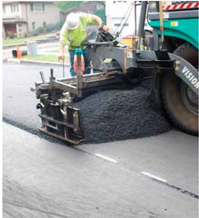
9.5-mm hot-mix asphalt Superpave is placed over the paving fabric. Photo courtesy of ISMF LLC.
