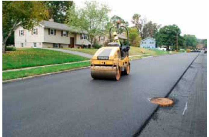
The Superpave mat is compacted prior to placement of a second pass. Photo courtesy of ISMF LLC.
