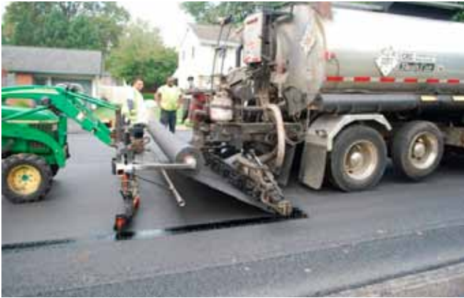
The paving fabric distributor truck sprays PG 64-22 sealant followed by placement of the paving fabric by the spreader/broom tractor unit. Photo courtesy of ISMF LLC.
