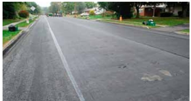
The paving fabric is placed over the Superpave leveling course, which was done the previous day to allow the roadway to cool prior to applying the sealant and paving fabric. Photo courtesy of ISMF LLC.
