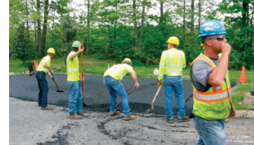
Warm-Mix Asphalt being applied in Patton Township, Centre County, as part of LTAP training in May 2013.
