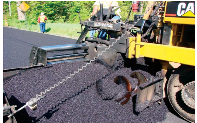
Warm-Mix Asphalt has no steam, thus improving working conditions at the paving site. The crew's first reaction was to say, "There's no smoke!"
