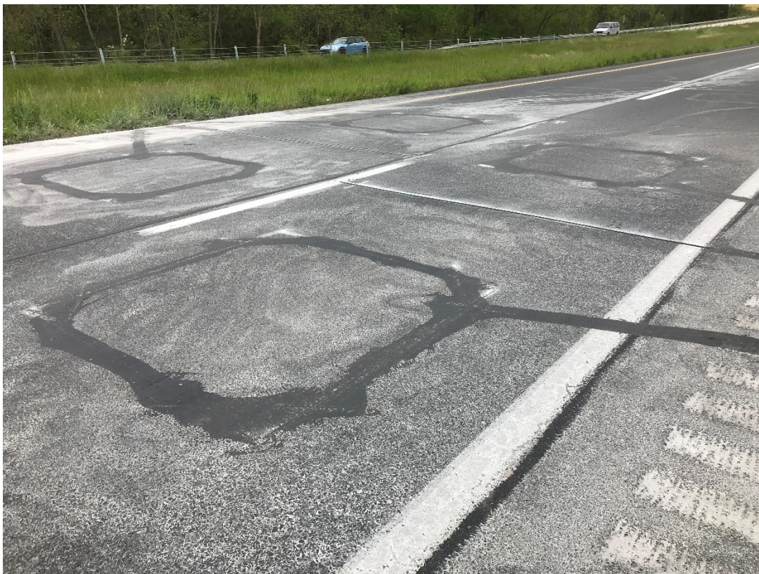
CAVC 848 Sensor Array on SR 15 in Adams County
