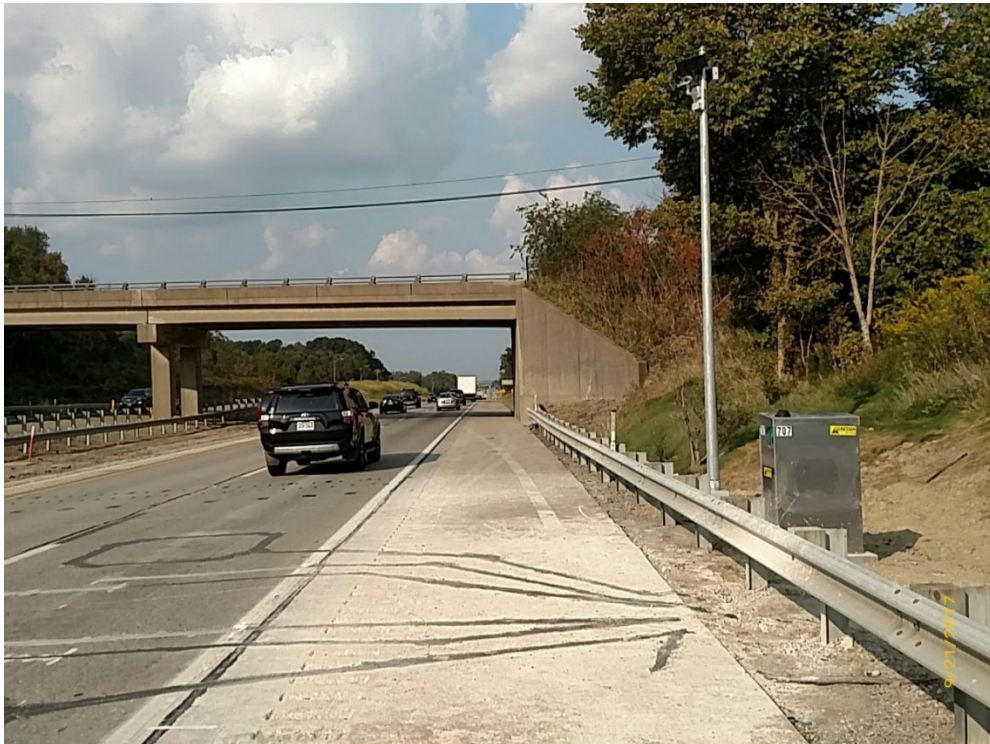
Completed installation of VWIM 707 in Allegheny County
