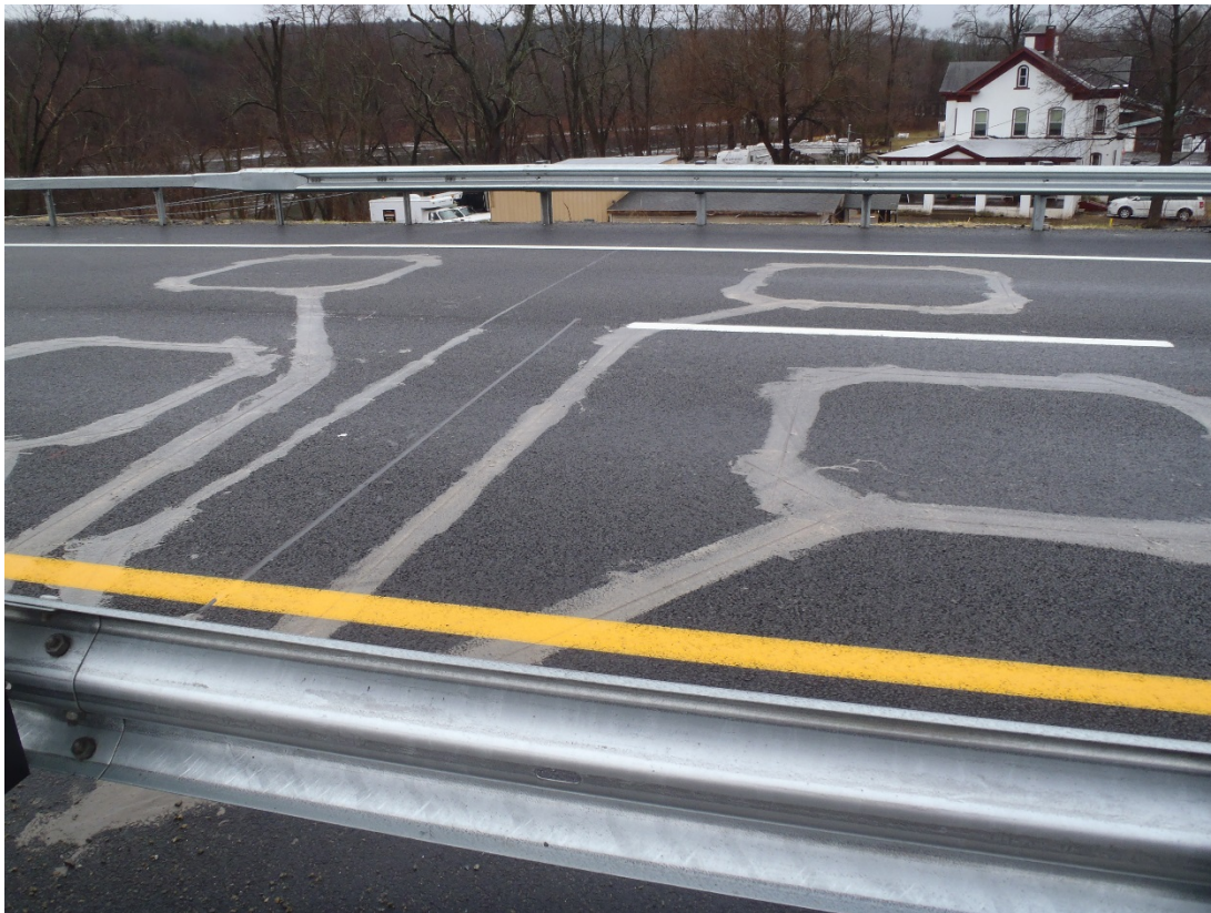
CAVC 818 Sensor Array on I-84 in Pike County
