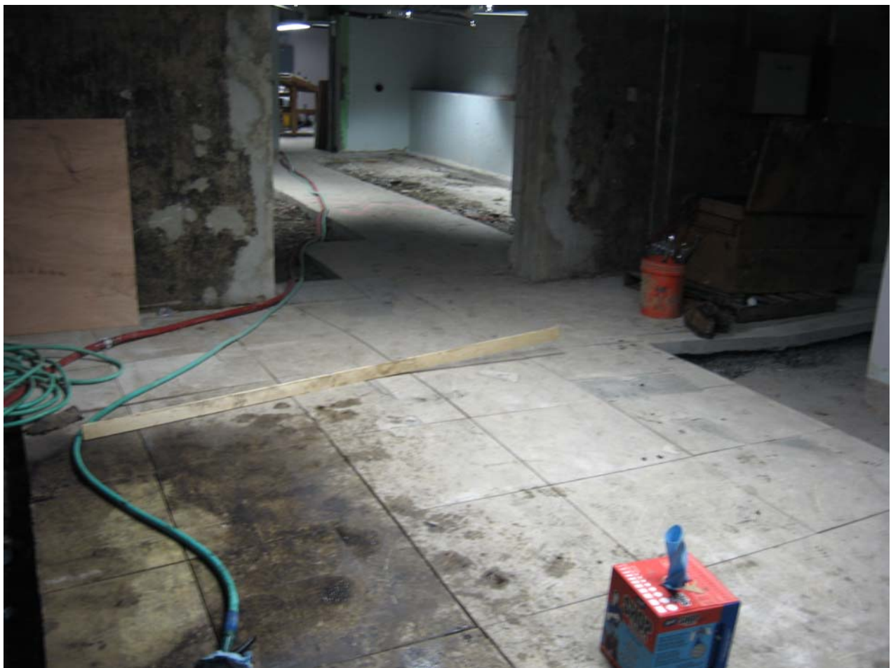
Figure 5.2. Visible heave of the floor slab built upon portions of the expansive Marcellus Formation at the Evangelical Hospital in Lewisburg, Pennsylvania.
