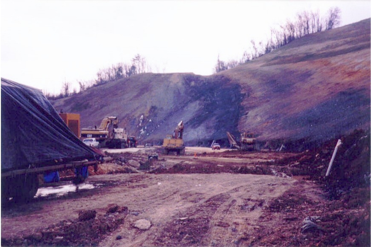
Figure 5.4. Photograph showing the black shales of the Marcellus Formation (center of photograph) exposed during construction along Route 522 west of Lewistown, Pennsylvania.
