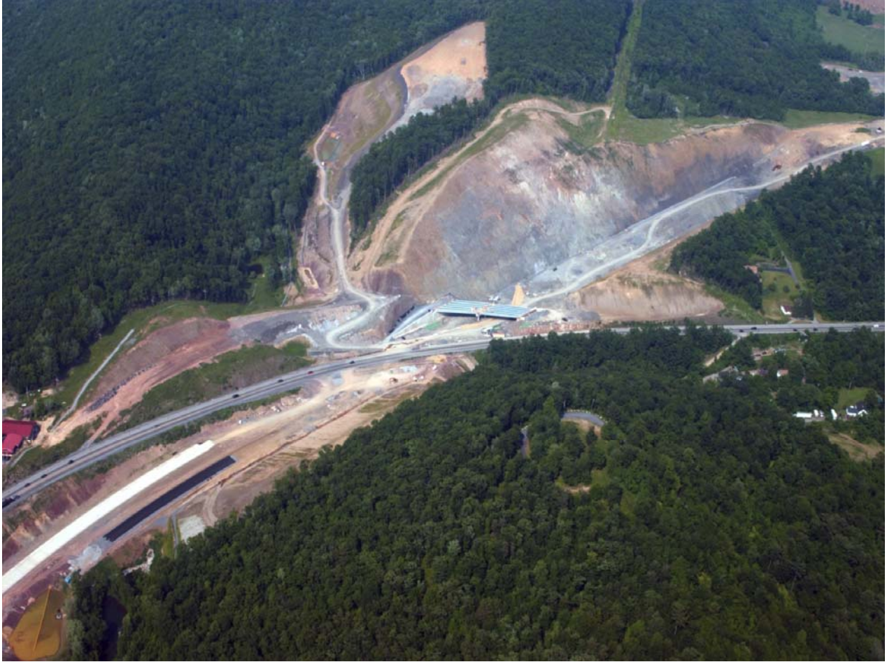
Figure 5.6. Aerial photograph of the main road cut at Skytop, Pennsylvania (D.P. Gold, Pers. Comm., 2007).
