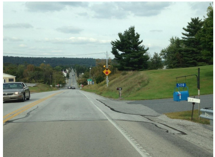
Placing longitudinal rumble strips along an edge line helps to increase safety although their use should be based on an engineering study.
