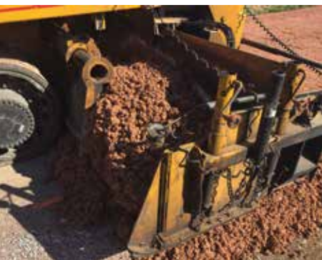
A paver is the preferred method for placing DSA on the subgrade.
