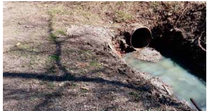
Leaking septic system adjacent to stormwater drainage pipe.
