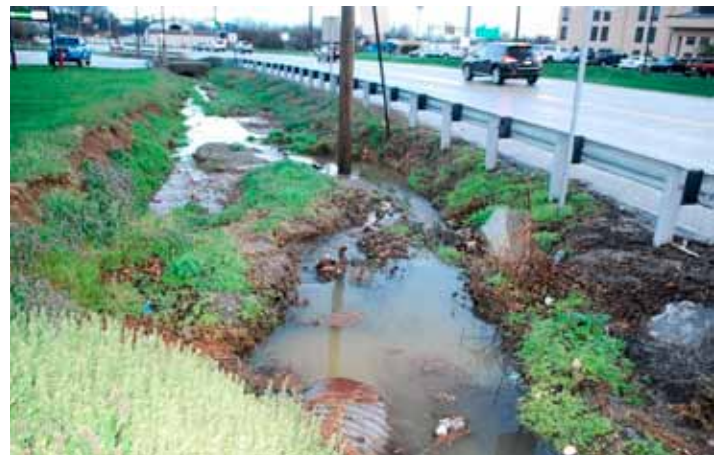
A municipal storm sewer outfall enters a stream that shows signs of contaminants.
